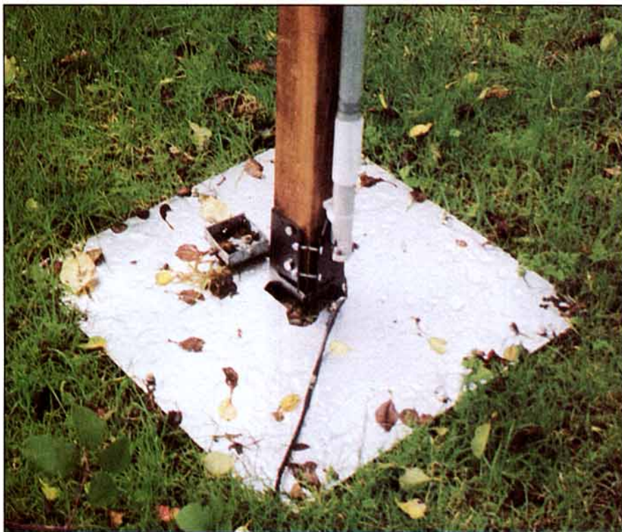
Base section of a vertical support showing the Metpost metal post support, vertical element fixed to the wooden post and the aluminium sheet section of the ground plane.
